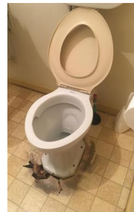
Damaged flooring in toilet Cracked toilet bowl
